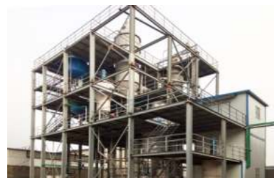
Wastewater evaporation crystallization system in the lithium battery industry
