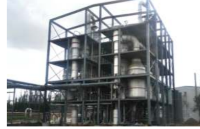
MVR sodium chloride evaporation system
