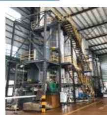
Desulfurized wastewater evaporation system
