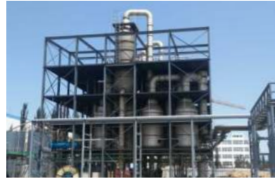
MVR sodium sulfate wastewater evaporation crystallization system
