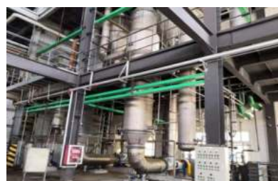
(Carboxymethyl)trimethylammonium hydrochloride evaporation crystallization system
