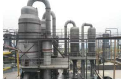
MVR ammonium sulfate evaporation crystallization system
