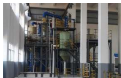
Nickel sulfate evaporation crystallization system
