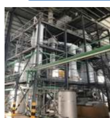
Sodium chloride wastewater evaporation system
