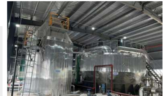
Ferrous Sulfate Continuous Crystallization System
